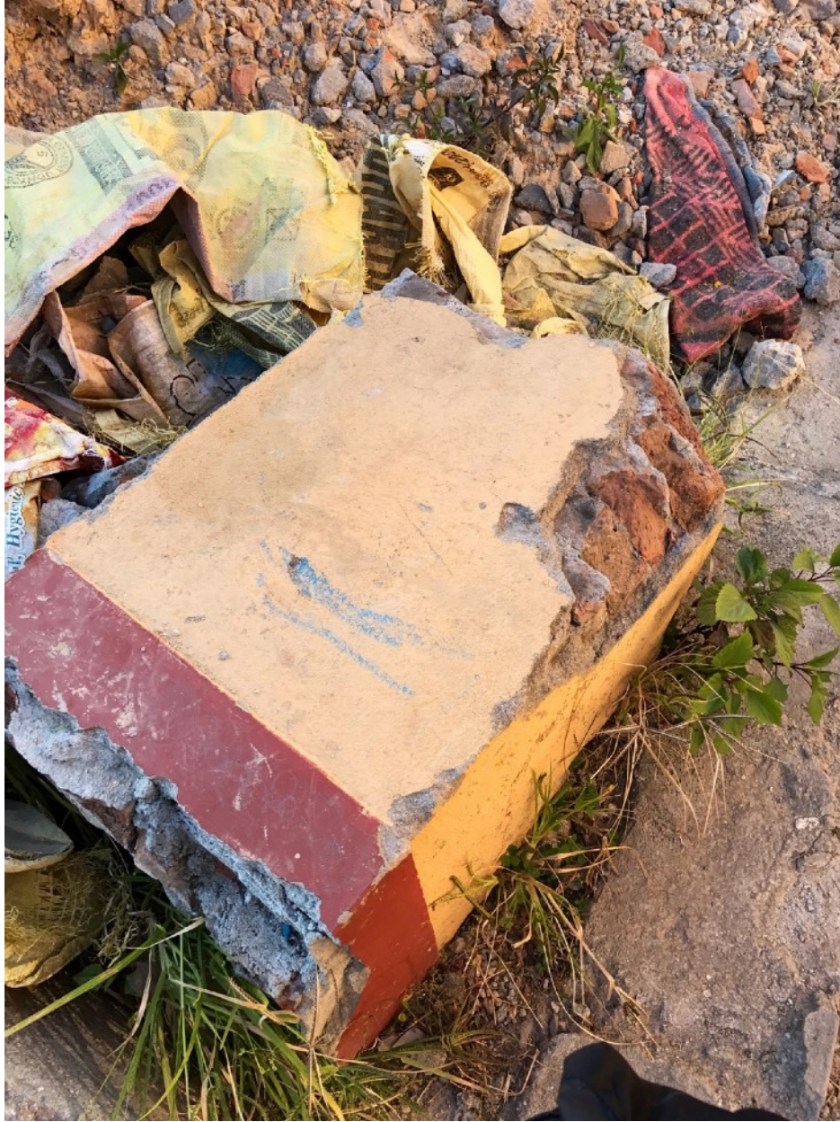
Pillar of monastery that was built on a mountaintop. Most of this monastery was damaged so severely it had to be removed and completely rebuilt. 建在山頂上的寺院柱子。這座寺院損壞相當嚴重，而需要移走廢墟，完全重建。
