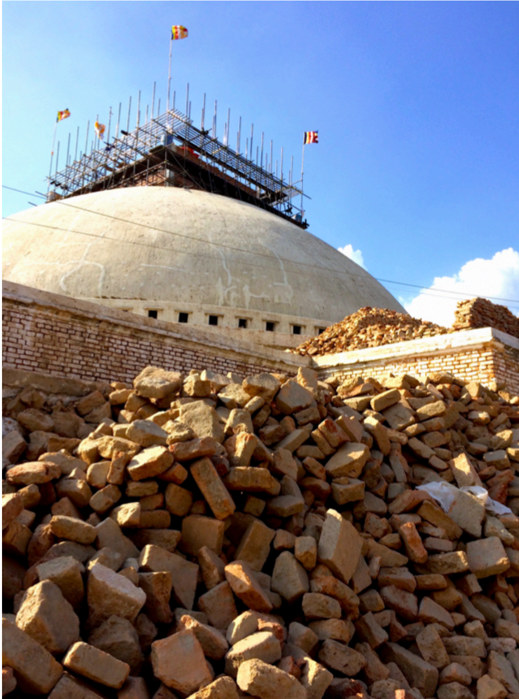
Rebuilding of Main Stupa in Kathmandu, amongst the rubble from the earthquake's destruction 加德滿都大佛塔在地震留下的碎磚瓦礫中重建
